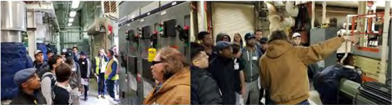
Keith Radich of the Central Chilled Water Facility explaining how the facility works and how PLC's are used to maintain the Chilled Water at a constant desirable temperature.
